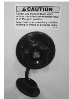
Tank Flush Inlet
